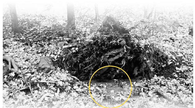
Spring (rust-colored water) that developed where the root ball of a tree pulled out of the ground near the downstream toe of a dam.
