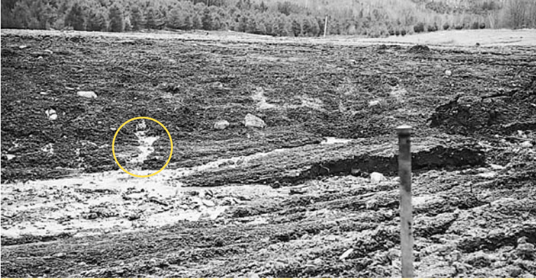
A spring discharging at the downstream toe of the embankment.
