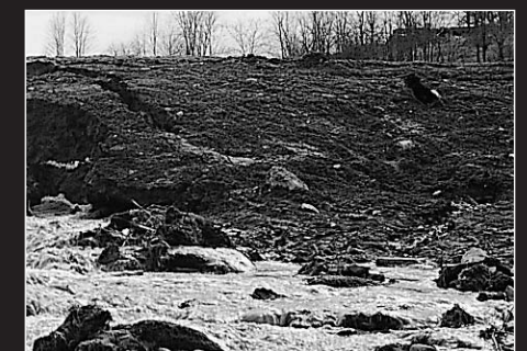
COVER PHOTOS Top: Shallow subsidence on the downstream slope of the dam. Middle: A cavity in the dam, revealed when the embankment was excavated with a back-hoe in the vicinity of the subsidence after the reservoir was lowered. Bottom: Close-up of the cavity, 6 feet wide and extending 85 feet into the embankment from the downstream toe of the dam.
