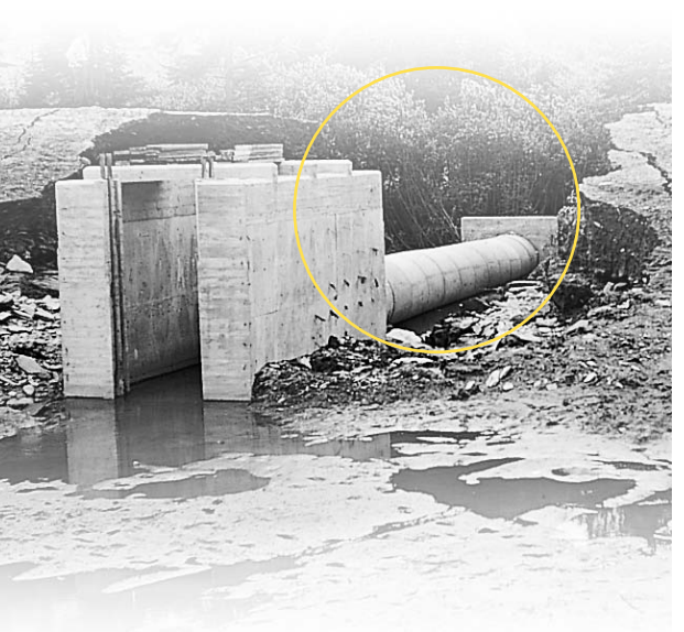
Failure of an earth dam by internal erosion along concrete outlet pipe.
