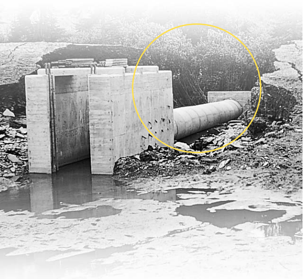
Failure of an earth dam by internal erosion along concrete outlet pipe.
