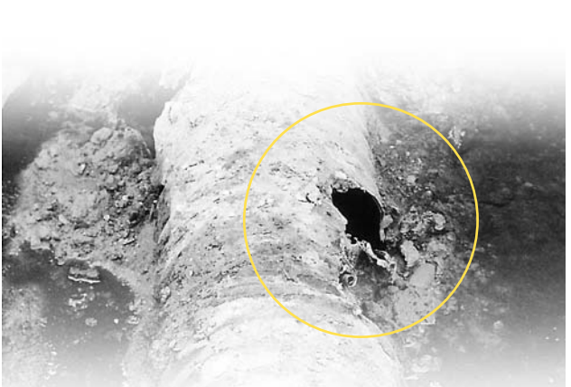
Corroded corrugated-metal outlet pipe removed from a dam that had developed large sinkhole.
