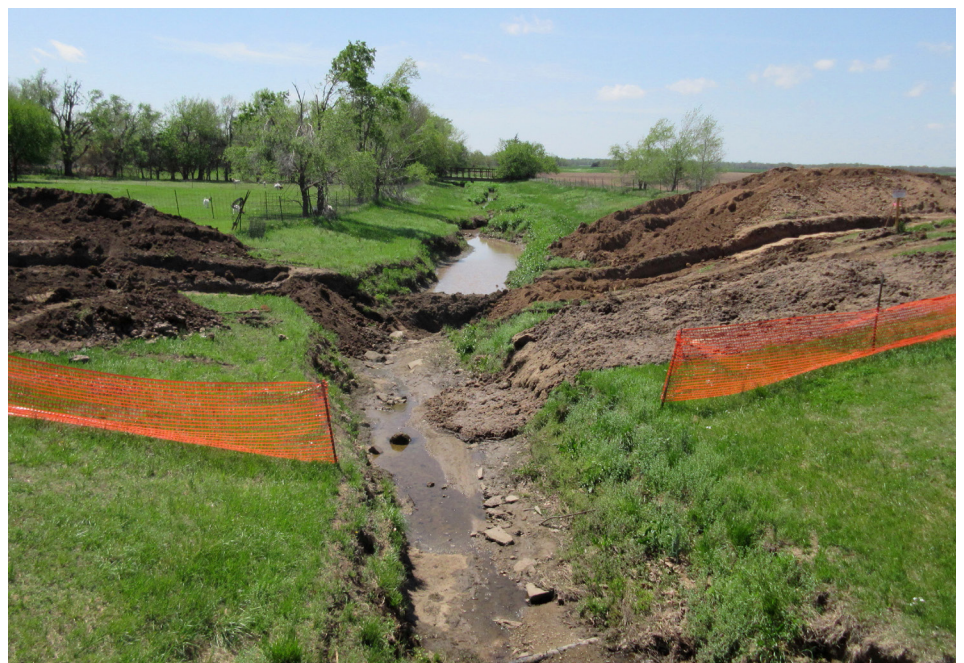
A trench has been dug across Salt Creek in Kansas, to install a pipeline. Improper management of spoils has led to silt impoundment within the stream bed, and soil stockpiles sloughing into the stream. Photo courtesy Steve Samuelson, Kansas Department of Agriculture.
