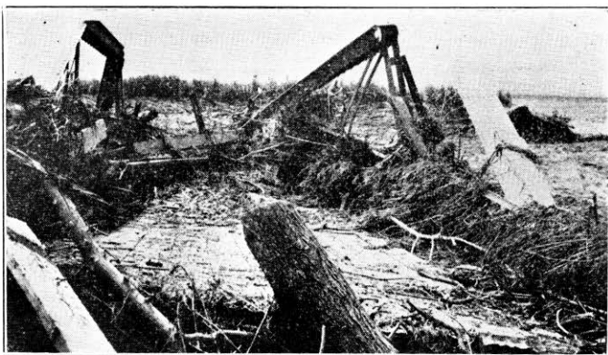
Typical damage caused by debris piling up against one of the older type bridges.
