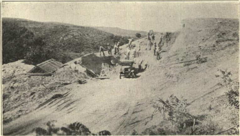
Loading a truck by hand shoveling on a drought relief project, on the Center-Bloomfield Road.
