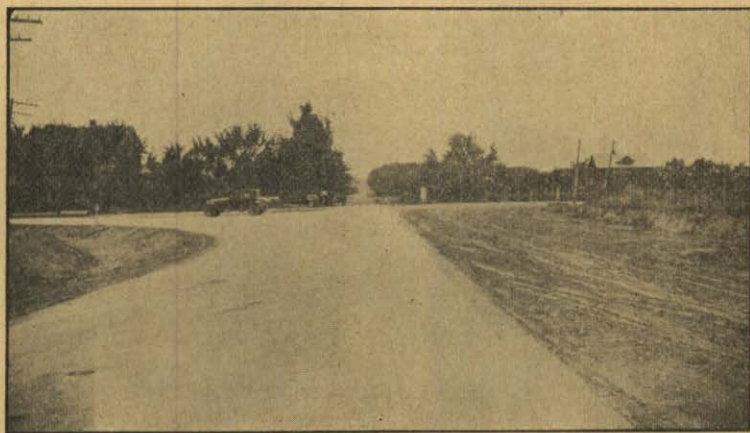
Lincoln County Project 221-A bituminous concrete pavement connecting North Platte and the State Farm.
