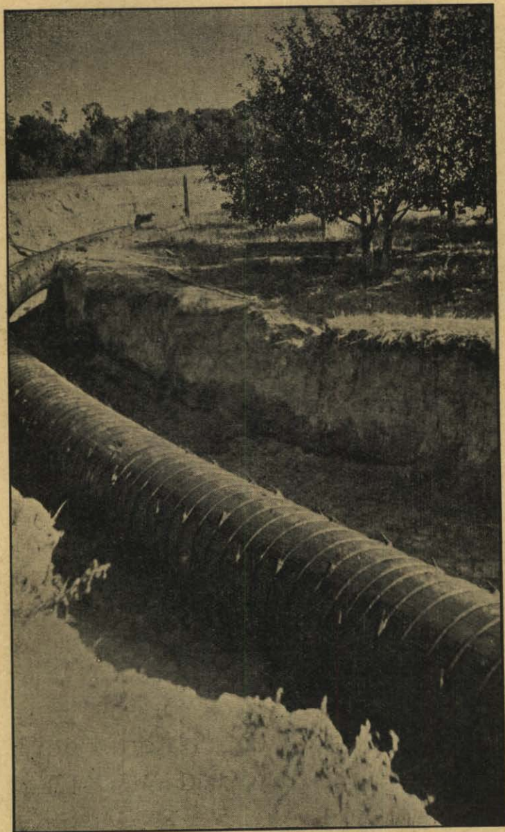
Pipe Line—Whitney Irrigation District
