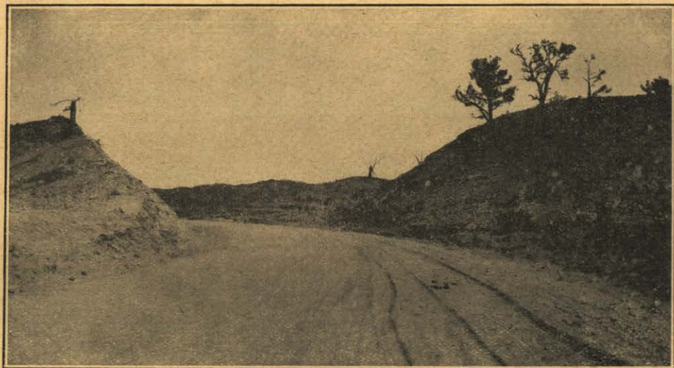
BERRY HILL APPROACH ON THE VALENTINE-SPARKS FEDERAL AID PROJECT NO. 66. Decreased Grade and View Ahead Provided By the Improvement. Note Width of Roadway and Depth of Cut.
