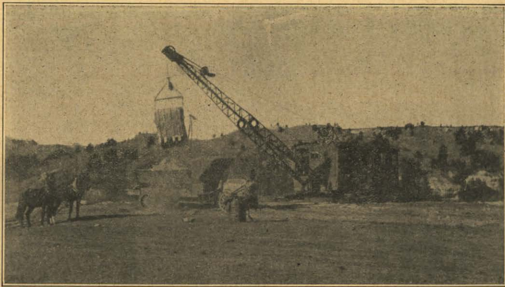
SOME OF THE EQUIPMENT USED IN CONSTRUCTING FEDERAL AND STATE AID PROJECT NO. 66, VALENTINE-SPARKS ROAD
