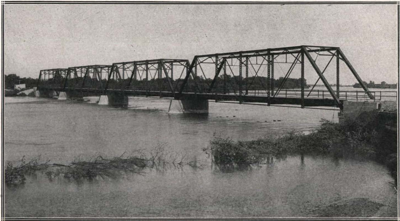
LOUP CITY STATE AID BRIDGE, MIDDLE LOUP RIVER. BUILT 1912, FOUR 120-FT. TRUSSES
