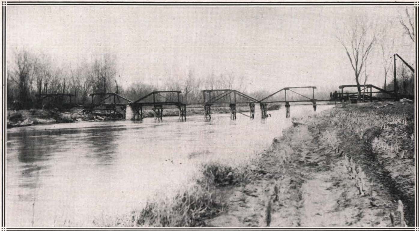
GRETNA STATE AID BRIDGE, DEC. 1, 1916. ELKHORN RIVER. UNDER CONSTRUCTION THREE 100-FT. TRUSSES
