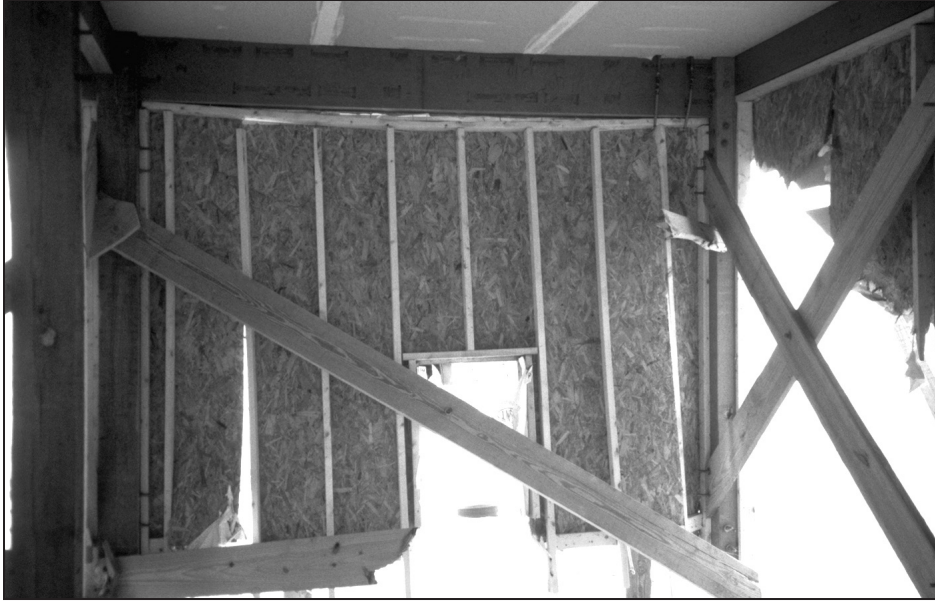
Figure 7. Non-compliant bracing arrangement
