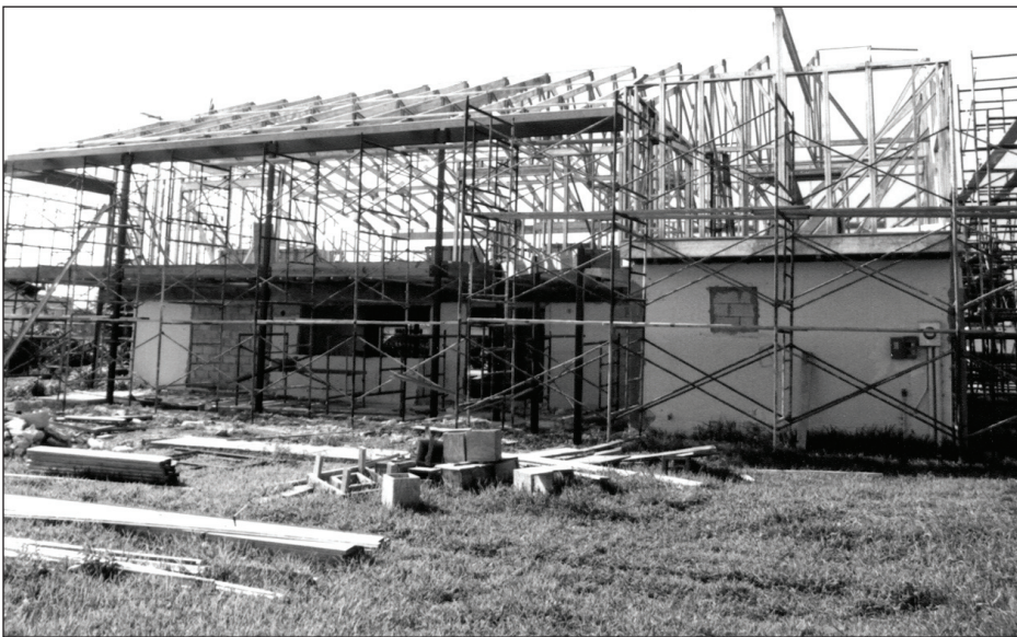
Figure 3-6. The owner of this flood-prone home in south Florida decided to build a new wood-framed second story on top of his masonry first story. The new second story is well above the BFE.
