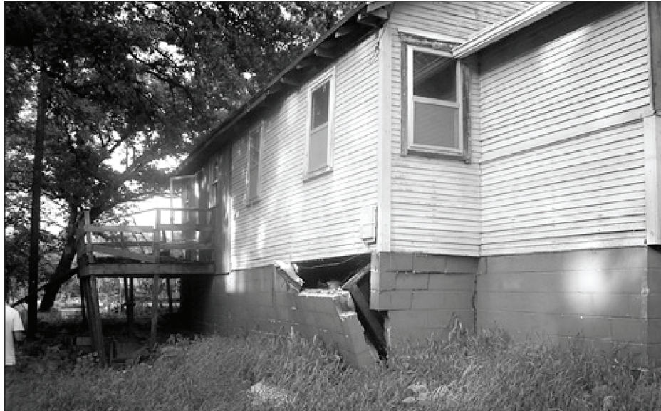
Figure 2-8. The walls of this basement in Iowa failed because of the pressure exerted by water and saturated soil.
