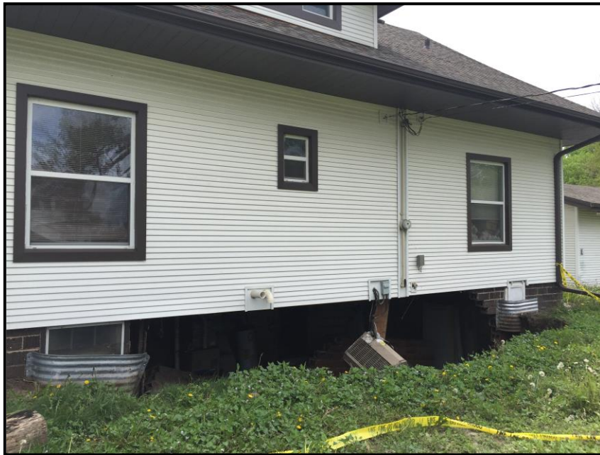
Figure 2. Home damaged from flooding in 2015 in DeWitt.
