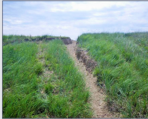
Dam embankment damaged by livestock.
