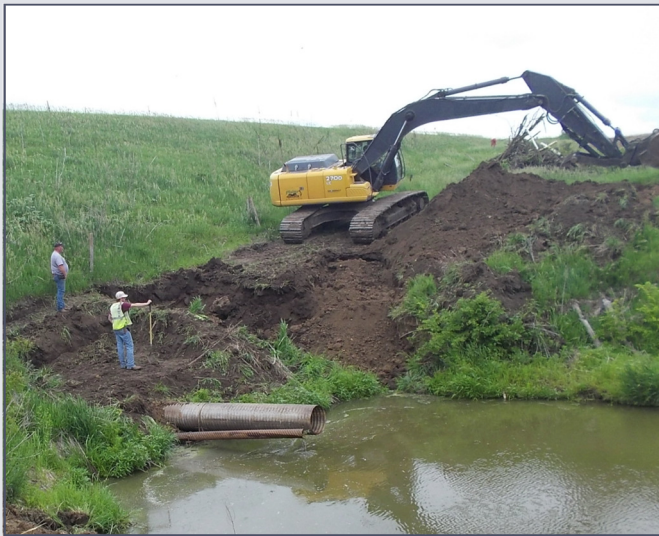
To repair damage, large rodent burrows may need to be excavated and backfilled with compacted soil.
