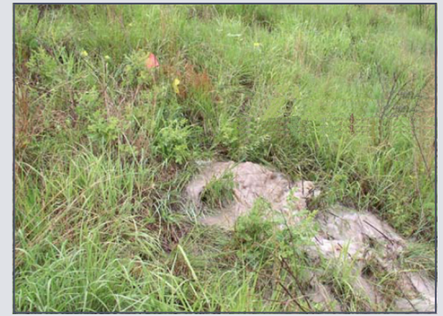
Cloudy seepage emerging from the downstream slope of dam in Frontier County, an indication that internal dam erosion was occurring. (Photo source: NRCS)
