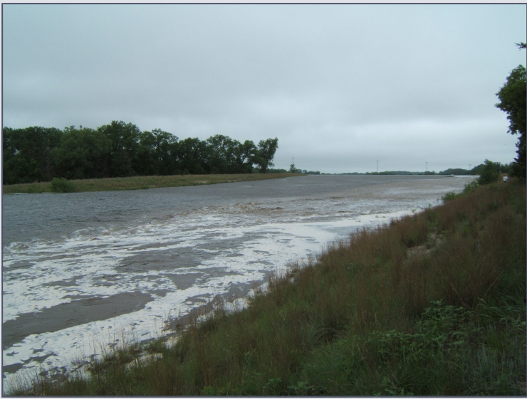
Auxiliary spillway flowing at a dam in Wheeler County. Spillways should be kept free of obstructions such as trees, posts, fence lines, and equipment that will catch debris and cause turbulent flow.
