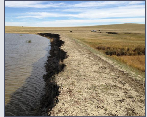
Failure to address erosion issues as they develop leads to costly repairs.
