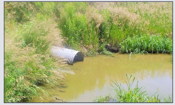
Standing water in outlet pipes accelerates corrosion of metal pipes and reduces spillway capacity.
