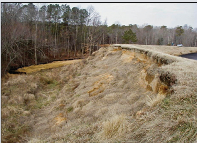
Large slide extending into the crest of a dam. Slides are typically caused by unstable steep slopes and saturated soil conditions following heavy rainfall. Slides can also be caused by rapid draining of the reservoir. (Photo Source: USDA)
