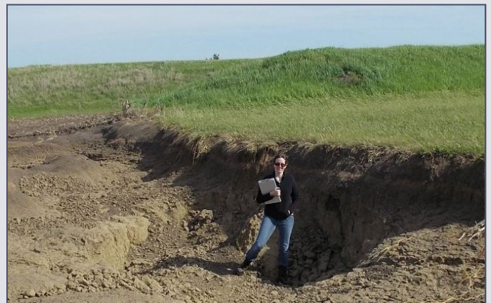
Erosion in auxiliary spillway where grass cover was removed and planted to crops.
