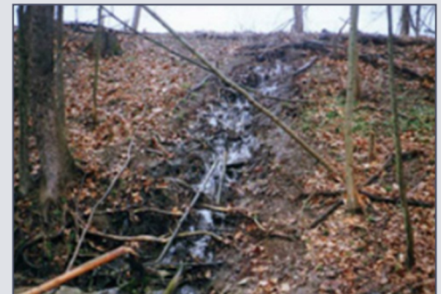
Seepage through dam damaged by tree roots. Trees should not be allowed to grow on dams. (Photo: ASDSO)
