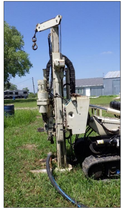
Photo shows a direct-push rig preparing for in-situ enhanced bioremediation injections into the aquifers beneath the Former Lincoln Air Force Base Atlas "F" Missile Site 1 in Elmwood, NE.
