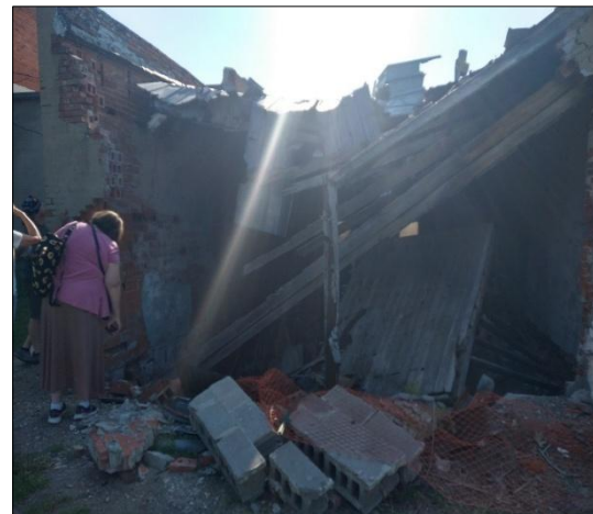
The Village of Upland shows NDEE, KSU TAB, and EPA the collapsed commercial building adjacent to their village office building during the Brownfields Resources Roadshow.
