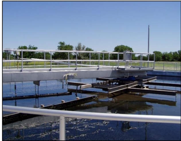
This photo shows a Wastewater Treatment Facility for Lincoln.
