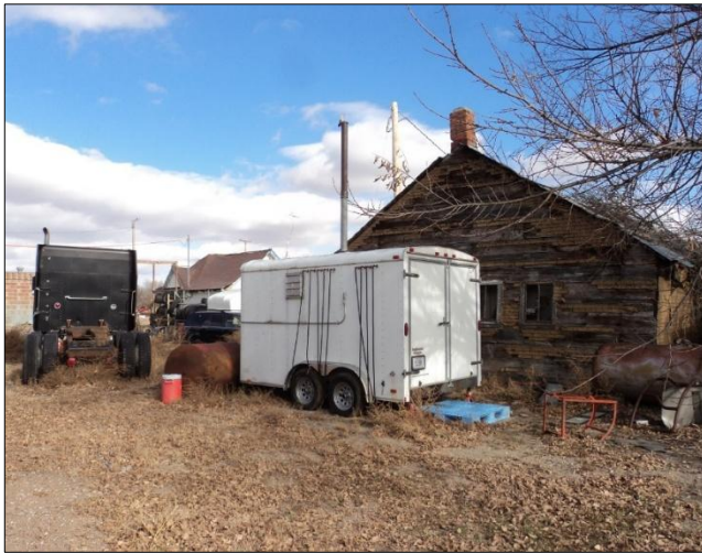
Air sparge/soil vapor extraction remediation system at the site of a former gas station.
