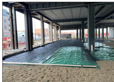
Vapor mitigation system granular layer and membrane
