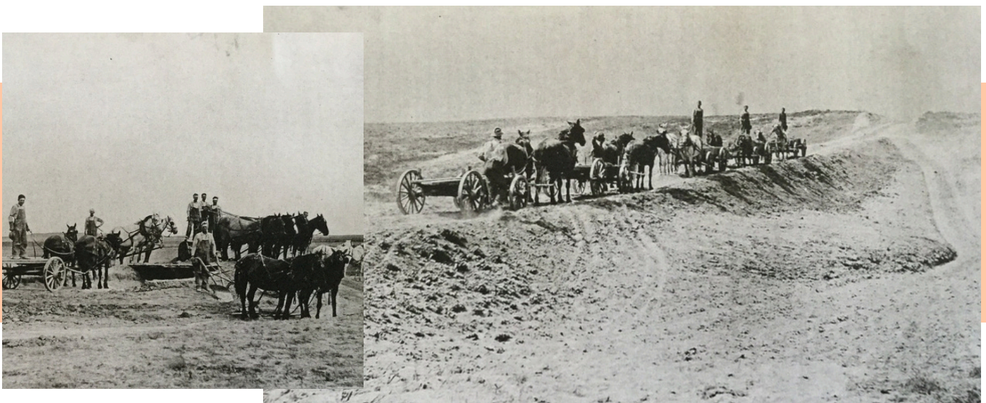
Work began on the canal in the 1890s. (Photos courtesy of Perkins County Historical Society)
